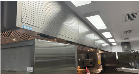
Kitchen hood supplied & installed
