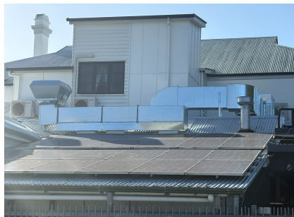
Kitchen exhaust & ductwork
