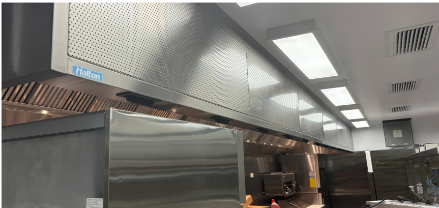
Kitchen hood supplied and installed
