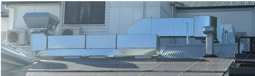
Kitchen exhaust and associated ductwork
